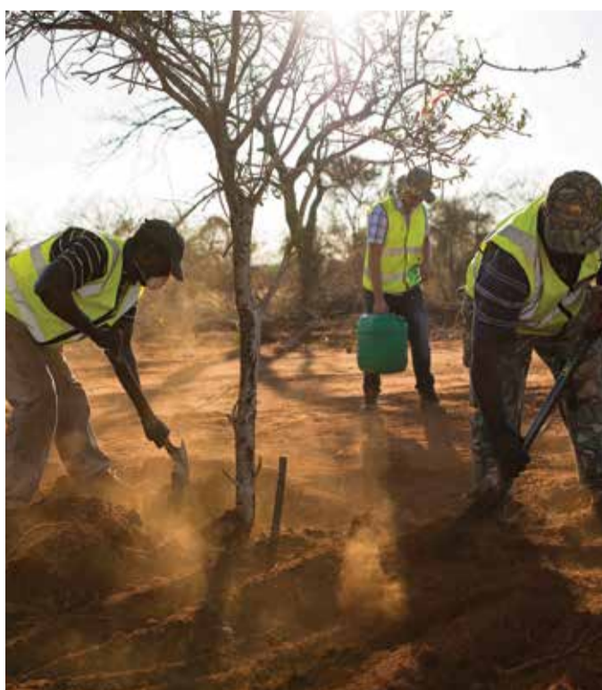
Relocation of one of many shepherd trees from the road reserved for the Musina bypass
